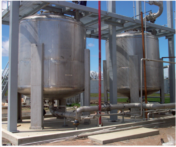
Mangere WWTP upgrade Fabricate and install, Stainless pressure vessels Water Care Ltd, NZ
